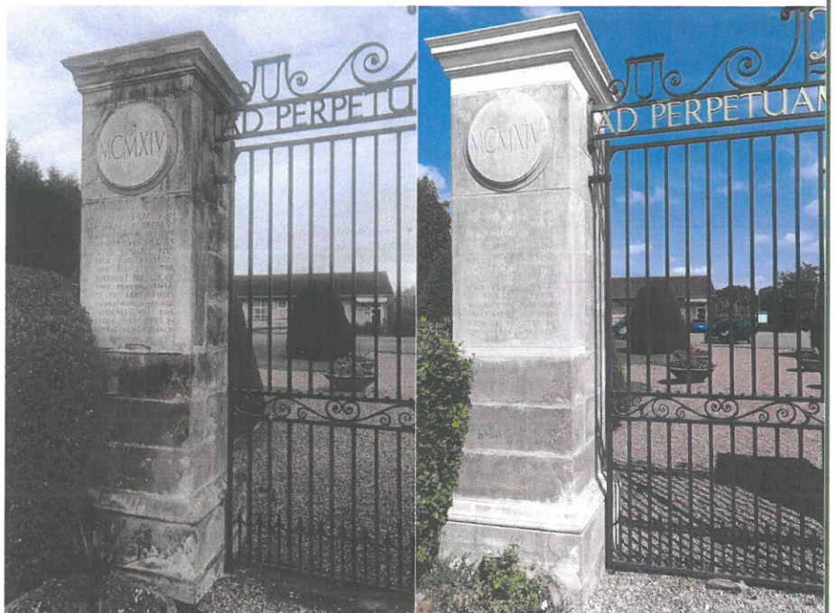
Above: Kirby Muxloe gates after works and below: pier before and after works (WM11506) © Kirby Muxloe Parish Council, 2021 and 2022
